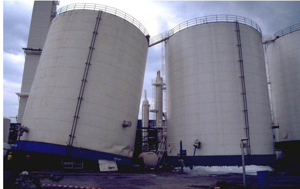
Plastic buckling of storage tank, 1999 Kocaeli earthquake (PEER 2000/09, Dec. 2000)
